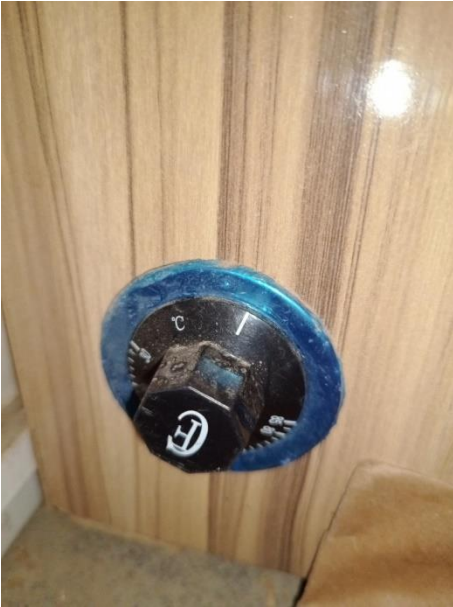
Fig. 3. The switch that is responsible for increasing the temperature of the whole system also serves as the switch for powering the whole system if the switch is on from the control box
